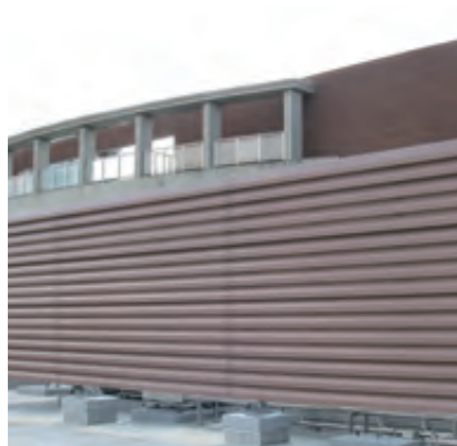
Noise control for an outdoor unit: facility in Osaka
