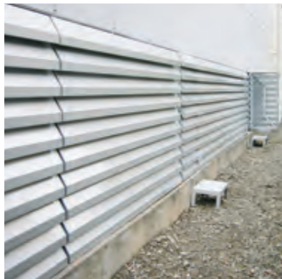
Noise control for an outdoor unit: electrical substation
