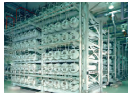
Reverse Osmosis Desalination Plant (RO)
