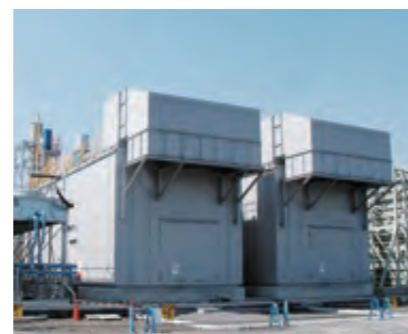
Noise control: gas engine enclosure
