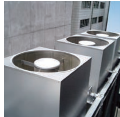
Noise control for an outdoor unit: facility in Tokyo
