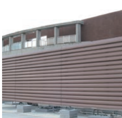
Noise control for an outdoor unit: facility in Osaka
