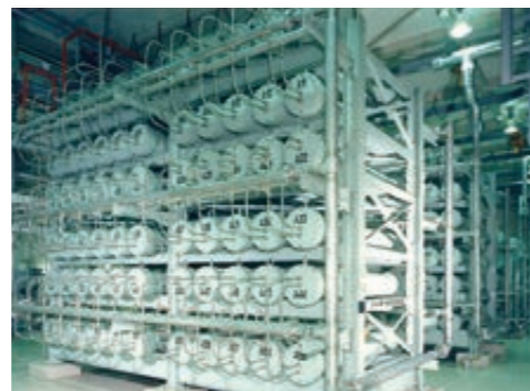
Reverse Osmosis Desalination Plant (RO)
